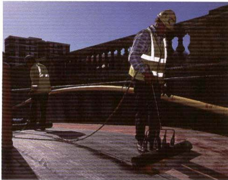
Photograph 9.1 — Torch-on roofing felt being applied to waterproof a concrete bridge deck. (Photograph courtesy of Cambridge Asphalt Co Ltd)
